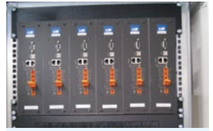
Control cabinet with motion controllers, monitoring system and master PLC
